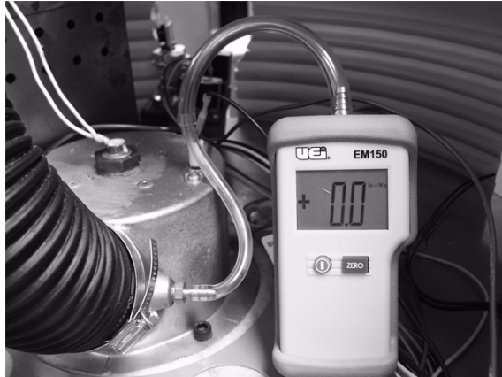
Blower prover and blocked outlet pressure
